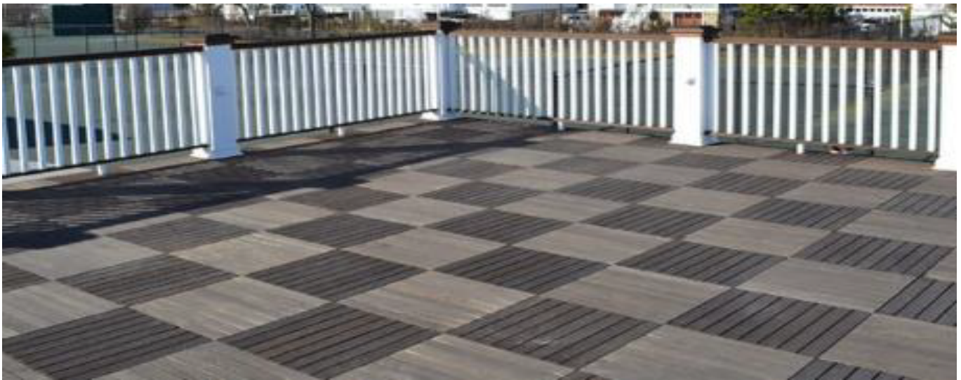
Weathered Deck Tiles
