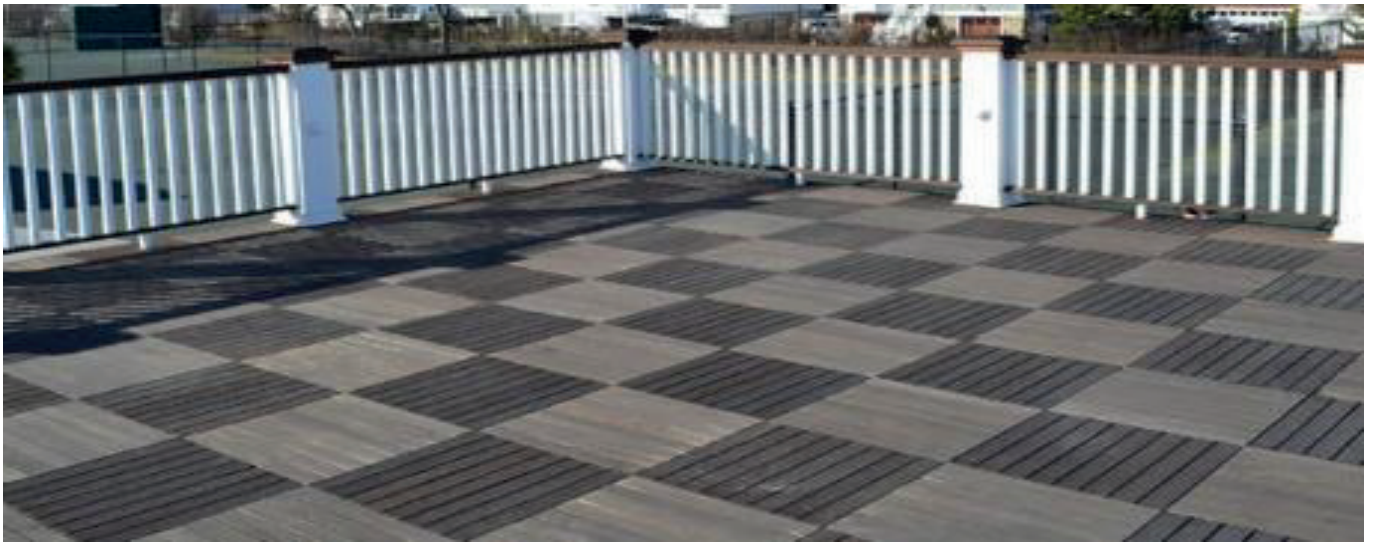
Weathered Deck Tiles
